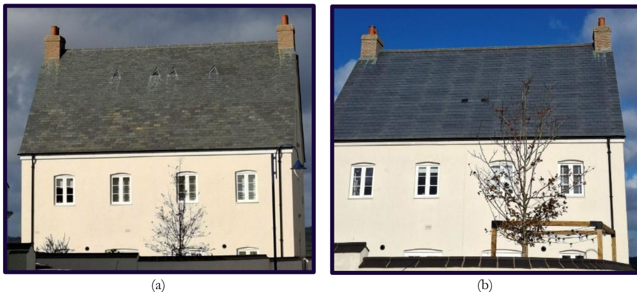
Figure 7: Nansledan: identical building design and roof typology showing (a) conventional roofing and (b) building-integrated photovoltaic (BIPV) roofing
