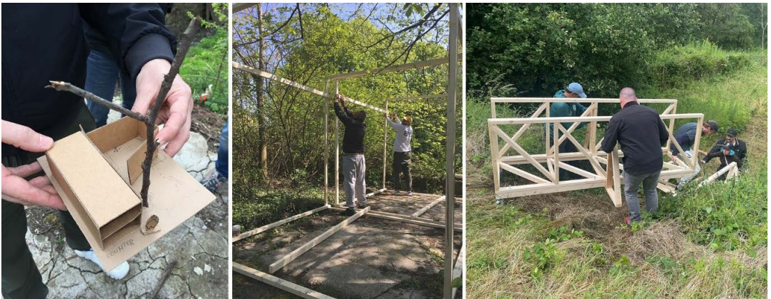
Fig. 4. Stefanescu. The Ripple Effect: Co-design workshops with stakeholders on site, utilising modelmaking, testing and 1:1 prototyping. 2023. Source: Author's own.
